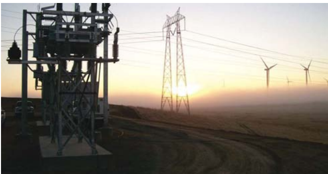
One of No. 3 Rosendin Electric's largest projects was the Shiloh II wind farm.
