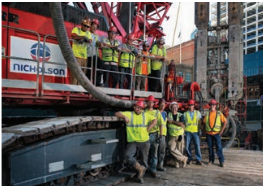
Nicholson Construction completed critical foundation elements of the bus ramp for the new $4.5-billion Transbay Transit Center in San Francisco.
